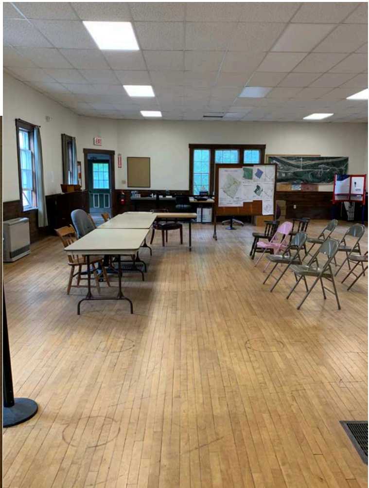
Upstairs common room (voting, committee meetings) Cannot be used for town meeting or community gatherings due to plumbing issues. Currently used by town Clerk during Covid to maintain social distancing
