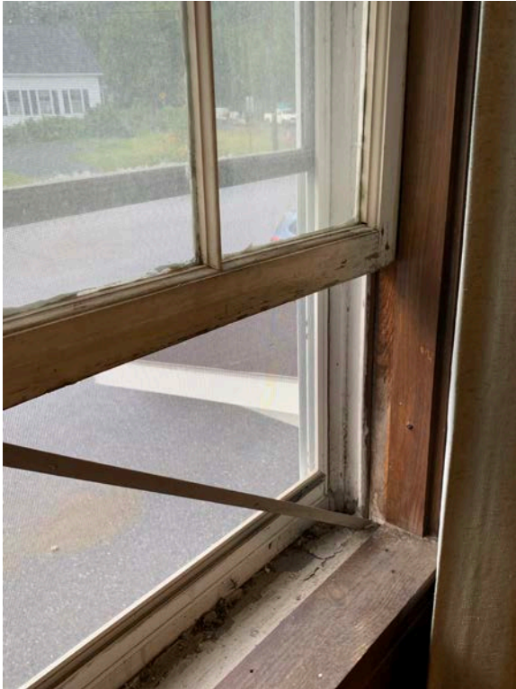
Older windows with storm and screen Are upstairs. Building has little to no Energy efficiencies
