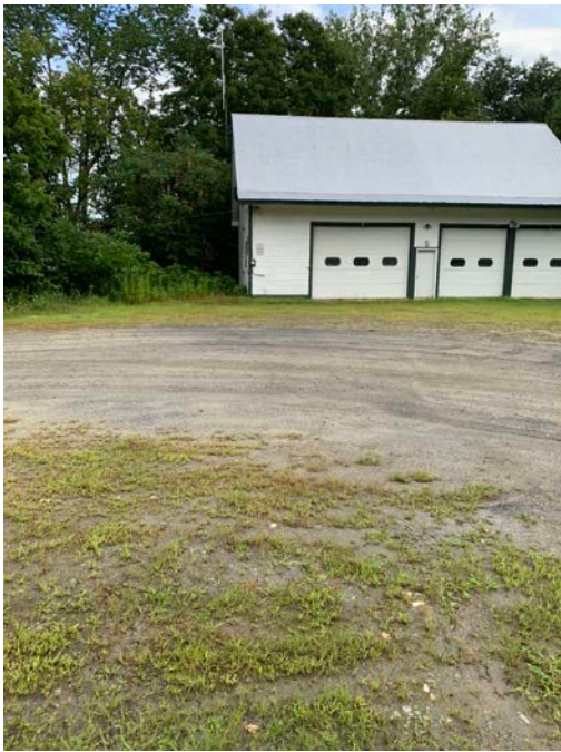
Parking circle behind back of building Leach field pipes frequently freeze and Cause plumbing problems in the building
